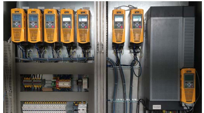
Fig. 1: Frequency controllers of the test bench. From left to right:
